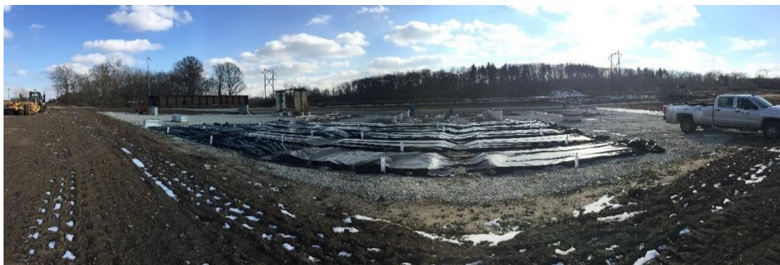
Figure 3-3: Panorama View of the Center for Aging Infrastructure: Slabs Covered for 28-day Curing
