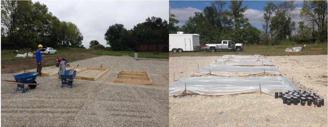
Figure 4-1: Pavement Form Installation for Mixture #1 at The Center for Aging Infrastructure Exposure Site (August 2014)
